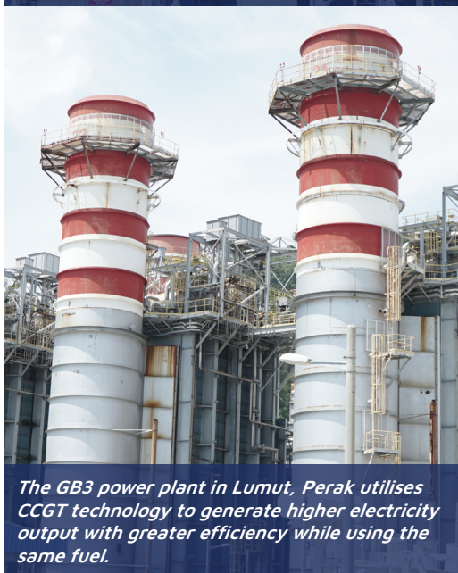
The SEV power plant in Lumut, Perak is the second largest IPP-owned CCGT plant in Malaysia.
