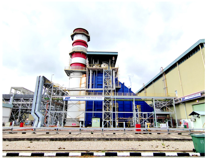
Segari Power Plant, Perak
